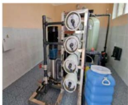
Photo 8. Functioning desalination equipment in Chimbay district
