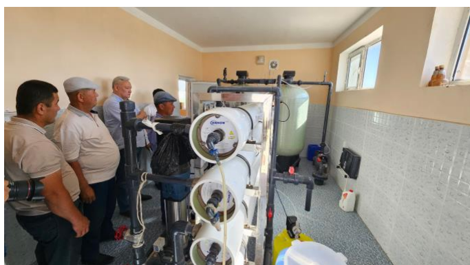
Photo 7. Water pumping equipment, Kegeyli district
